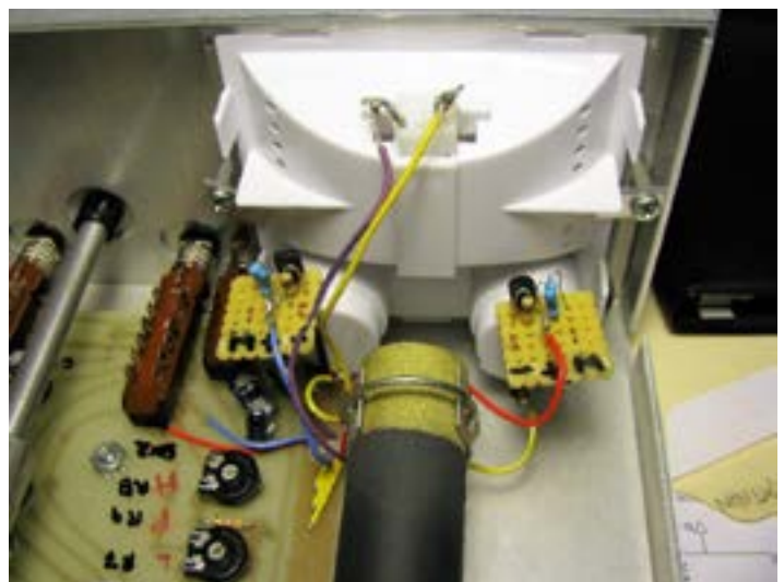
Figure 6. Limiters installed on back of meter movements
